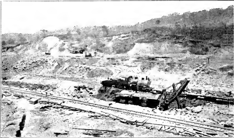
LAS CASCADAS SLIDE, CULEBRA DIVISION, APRIL, 1908. AREA OF SLIDE, 5,433 SQUARE YARDS. Estimated amount of material in motion, 100,000 cubic yards. This slide started in the dry season and extended back 230 feet from the edge of cut and to within 50 feet of the crest of the hill.
